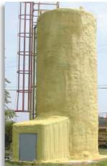
This water tank that supplies an automatic sprinkler system is protected from freezing by a combination of spray-on insulation and immersion heaters.
