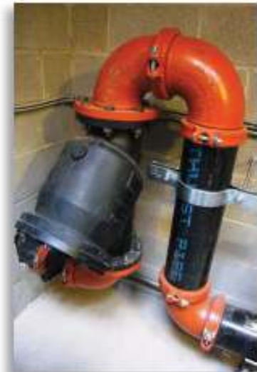
This inline strainer assembly is intended to protect a fire pump from damaging debris.
