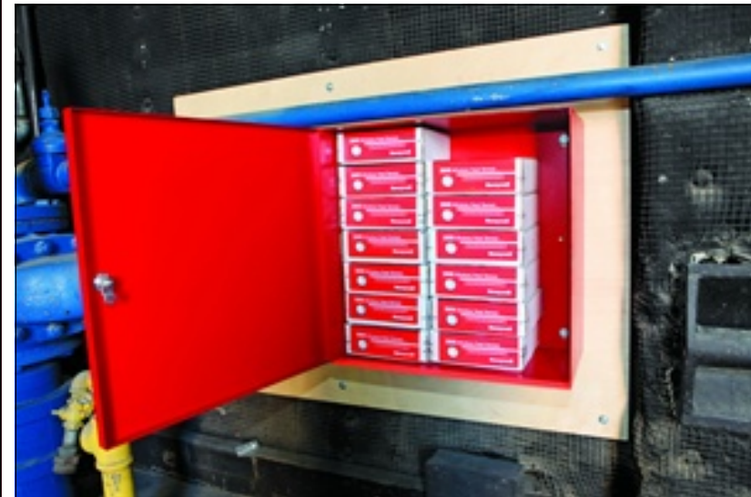
Each studio stocks wireless heat detectors that are programmed for the individual fire alarm control panels.
