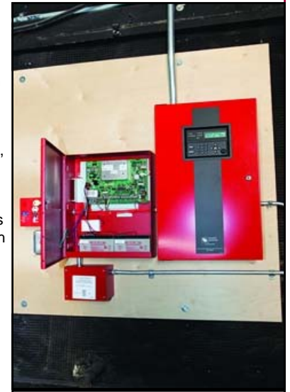
The sound stages had previously been outfitted with the Silent Knight 5207 conventional fire alarm control panel (FACP). In some instances, a single panel had been
