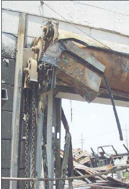
This fire door assembly failed during the Super Sofa Store June 18, 2007 fire. Photo courtesy NIST Building and Fire Research Laboratory.
